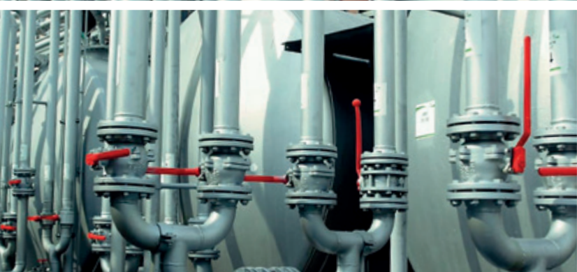
Ventilsystem im Tanklager The valve system of the tank storage
